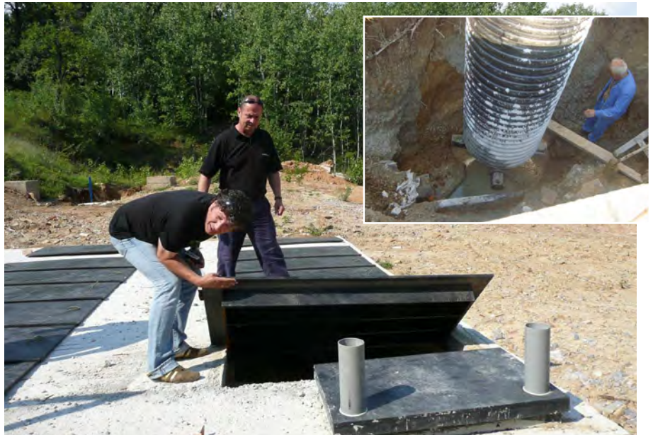
David Hollands and Julian Georgiev enjoying the final checking of the biological 'live bacteria' installation. Inset picture: One of the main inspection chambers being installed deep underground.
